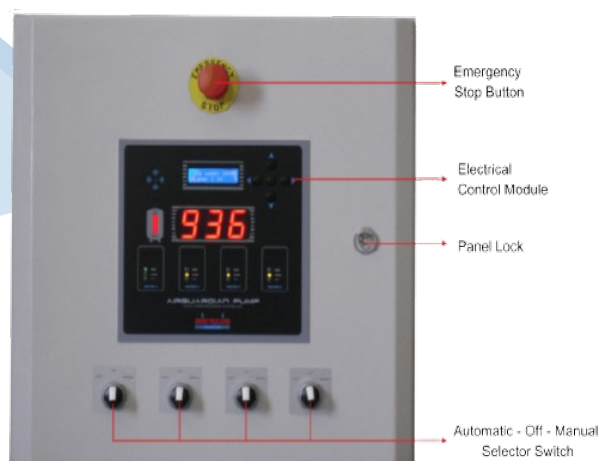
Front View of the Control Panel
